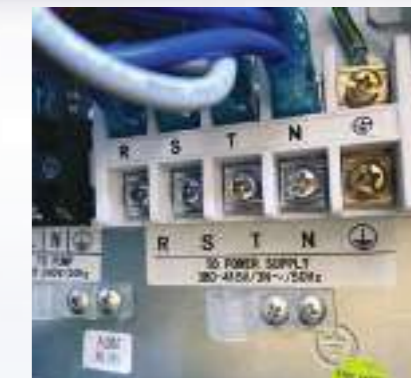
Power connection 3 fase (3)
