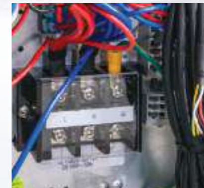
Power connection 1 fase (2)
